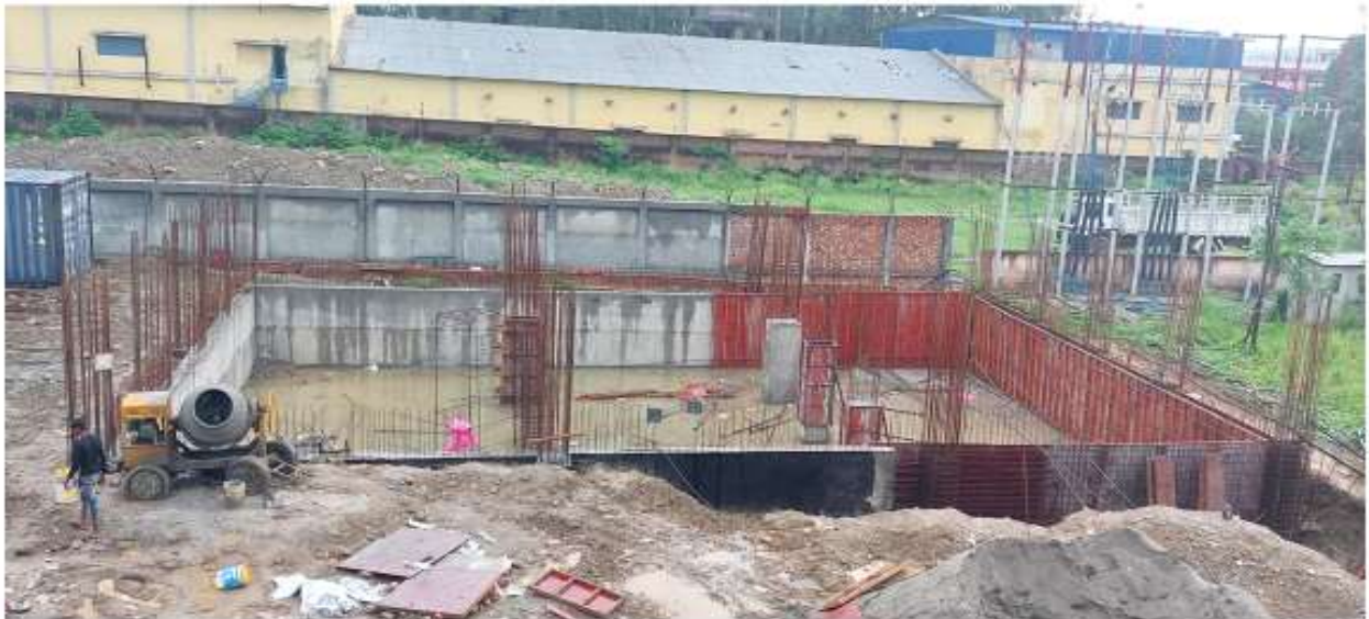
220 kv GIS Hall
